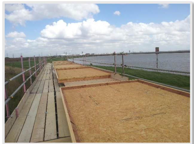
Wooden frames constructed as a base for the ephemeral wetland green roof experiment - Barking Riverside, London, UK. (©UEL SRI)
