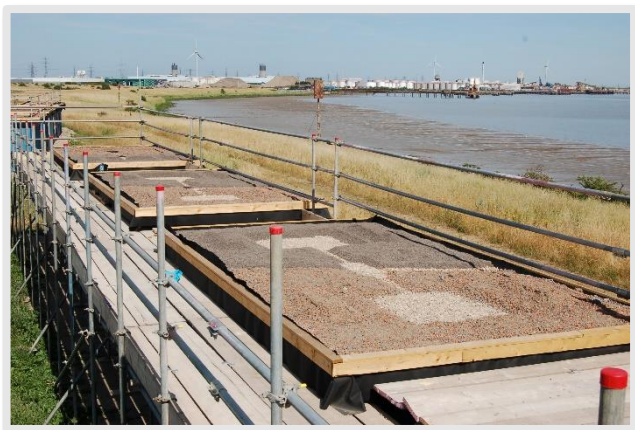
Freight containers with ephemeral wetlands green roofs with substrate installed. Barking Riverside, London, UK. (©UEL SRI)
